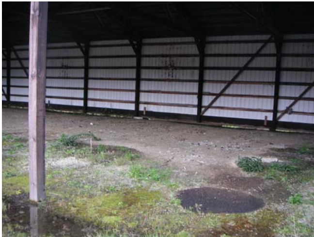
Photo 9: Staining in Bus Barn
