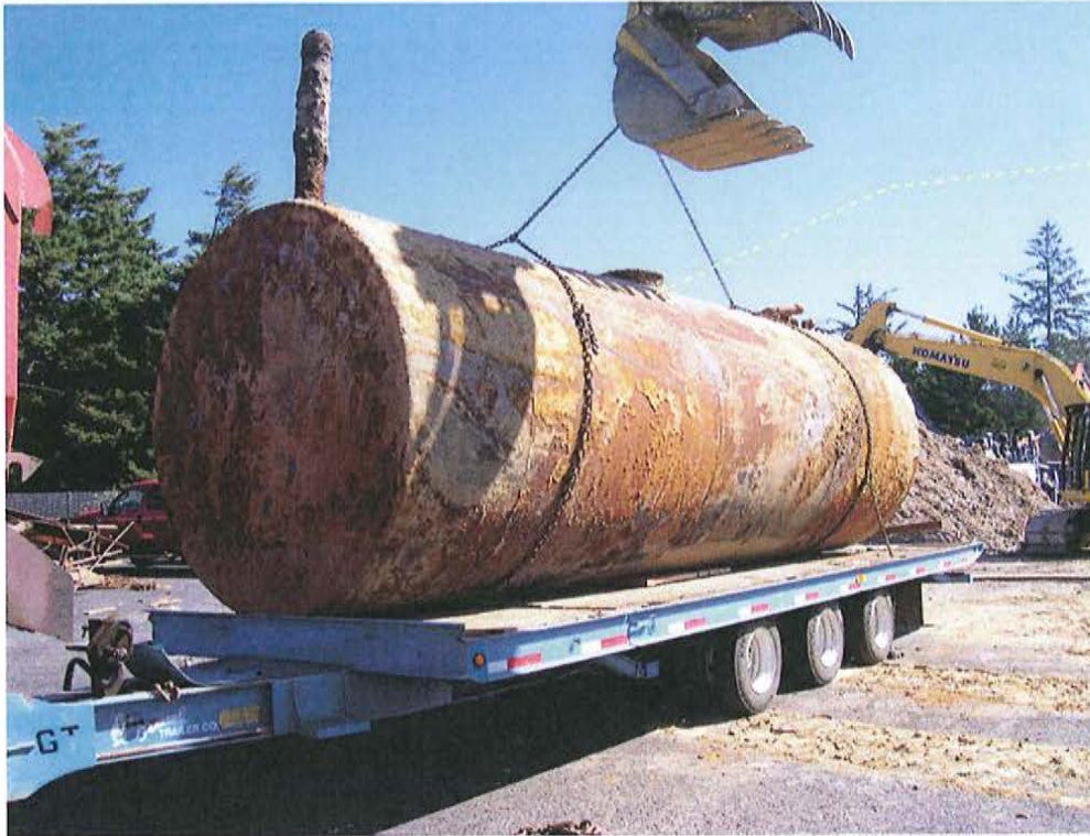
Photo 3: Tank removed and placed onto flatbed trailer for disposal. Tank observed in good condition with no visible signs of leakage or failure.
