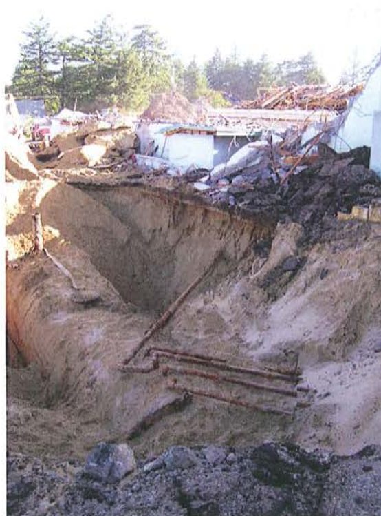
Photo 2: Looking northeast of one vent and four product lines.
