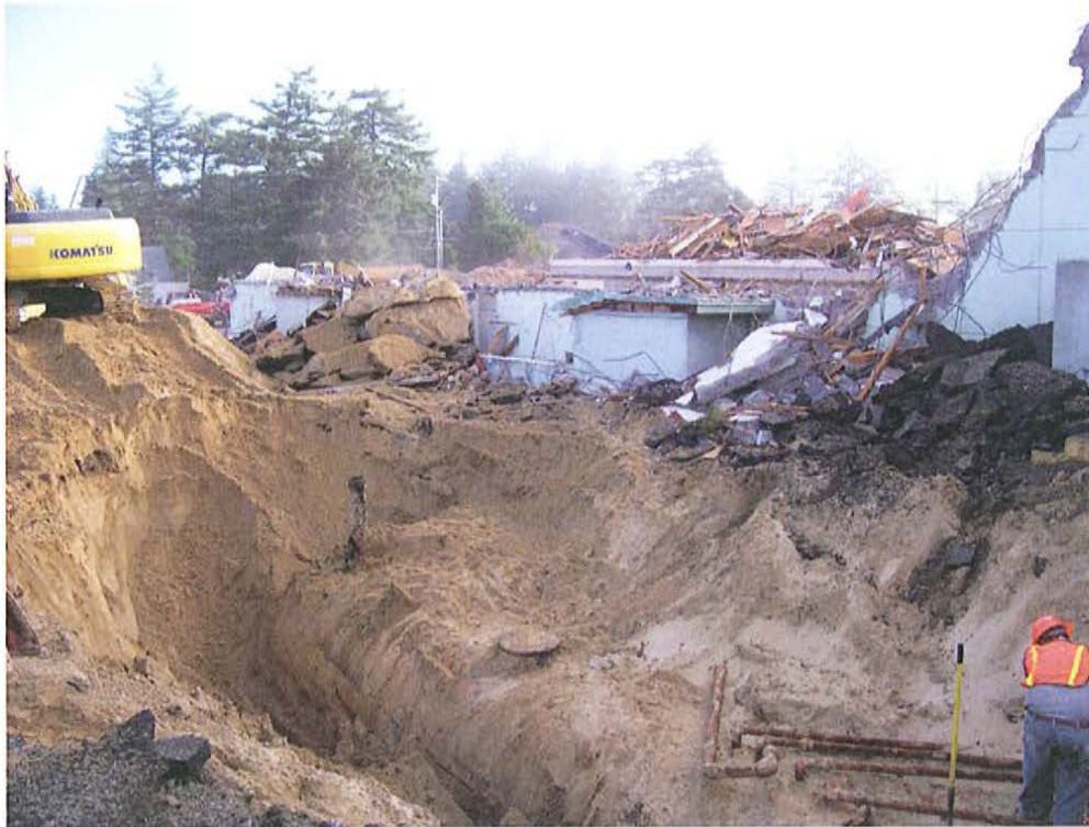
Photo 1: Looking northeast of unearthed heating oil tank. Tank, fill port, product and vent lines can be seen.
