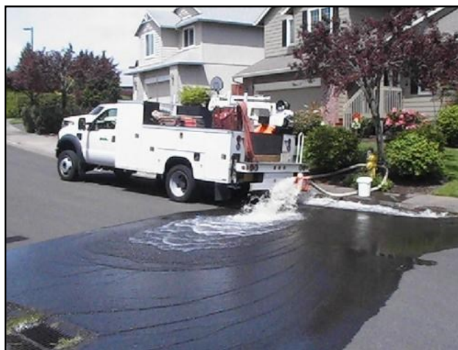
Water Distribution Crews flush hydrants on an annual basis to make sure they are working correctly.
