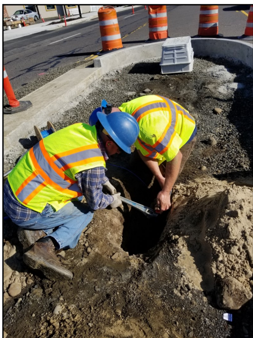
The City of Florence Public Works Department installs and maintains the water pipes that bring water to your home.
