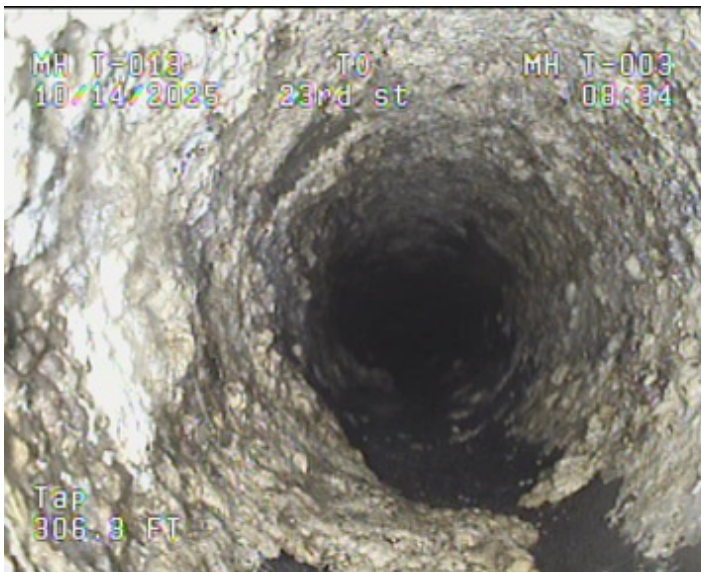
Sewer Pipe full of FOG
