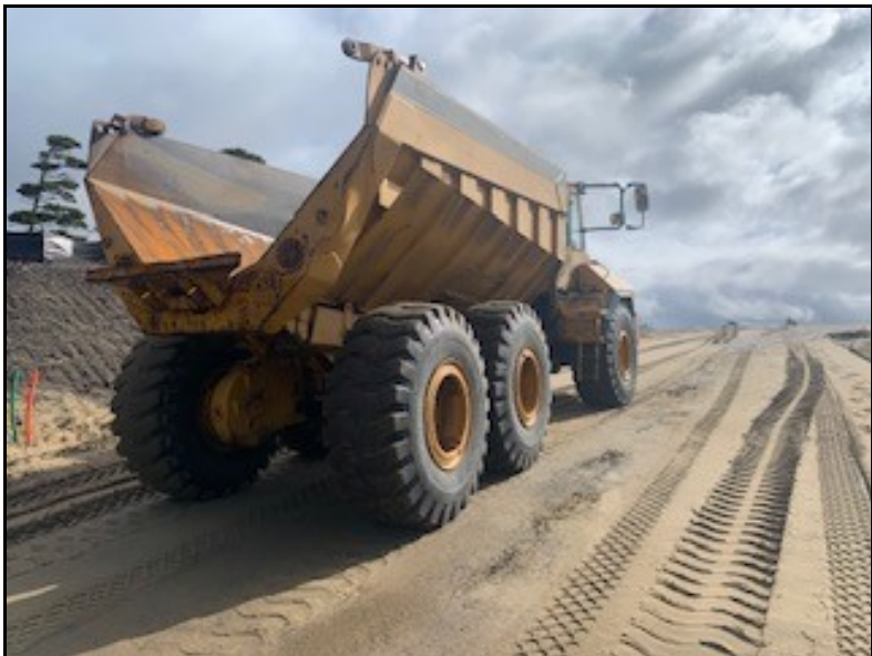
Photo 1: Looking east at the proofroll being conducted using the Moxey MT30 articulating tandem axled dump truck. This section of roadway is at the approximate 12% grade off North Rhododendron Drive.
