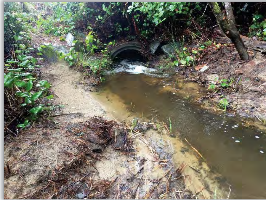
Figure 4-35 - 42-inch concrete culvert inlet, heavy sedimentation, evidence of exceeded capacity
