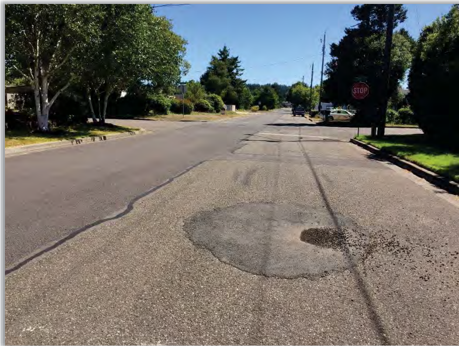
Figure 4-38 - Sinkholes forming directly above drainage lines. Evidence of pipe failure.
