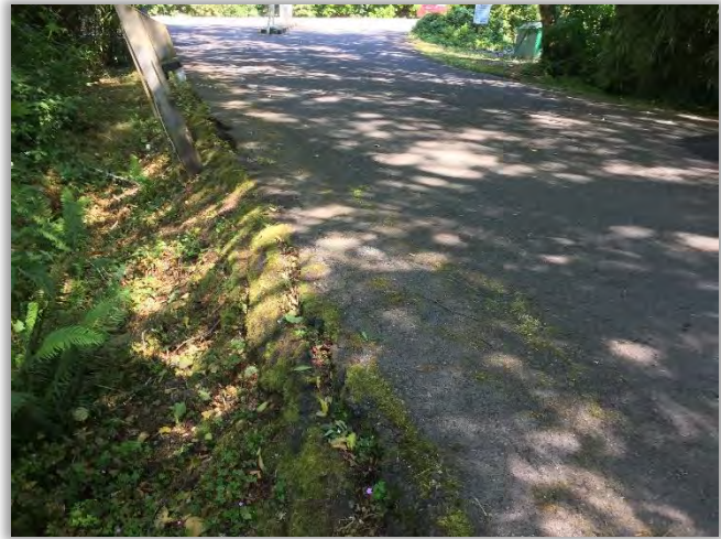
Figure 5-12 - Erosion at the roadway edge, steep slope, 31st Street, North side
