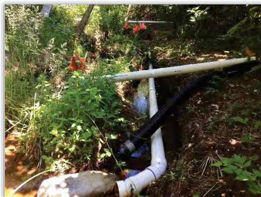
Figure 4-36 - Private drainage piping discharging into ditch. Efforts made by Seabrook Townhomes residents to alleviate flooding
