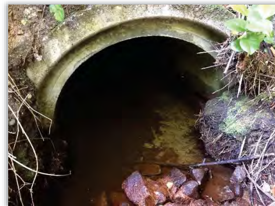
Figure 4-37 - Dry-season field inspection photograph of 42-inch concrete culvert inlet, silted in
