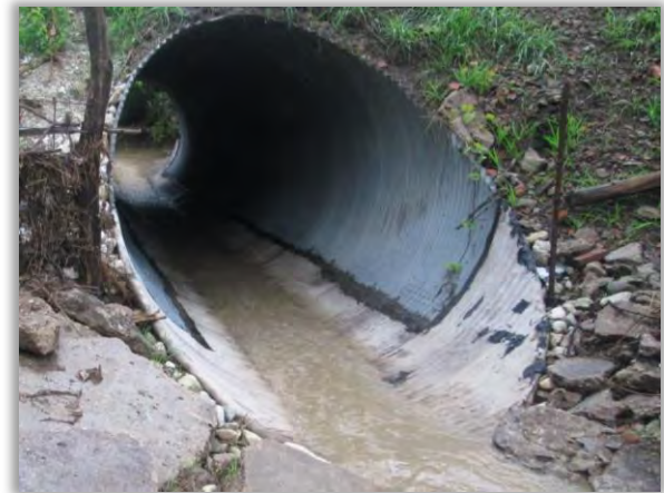
Figure 6-27 - Geosynthetic cementitious composite mat applied to CMP culvert to extend lifetime of culvert (example)
