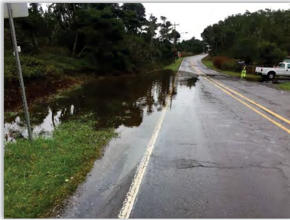
Figure 4-23 - Flooding on Rhododendron Drive
