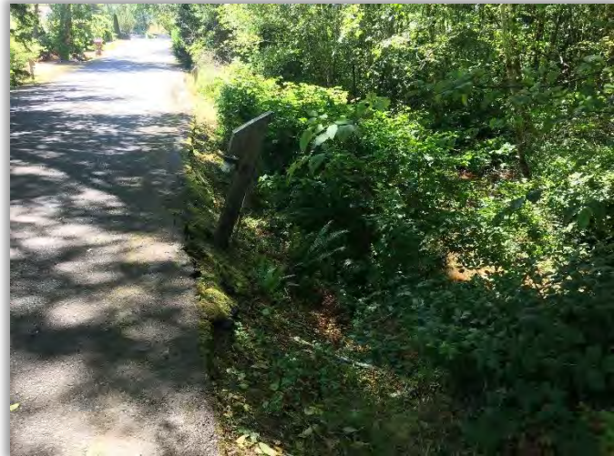
Figure 6-28 - Eroded edge of pavement. Address by replacing/extending culvert and adding fill material
