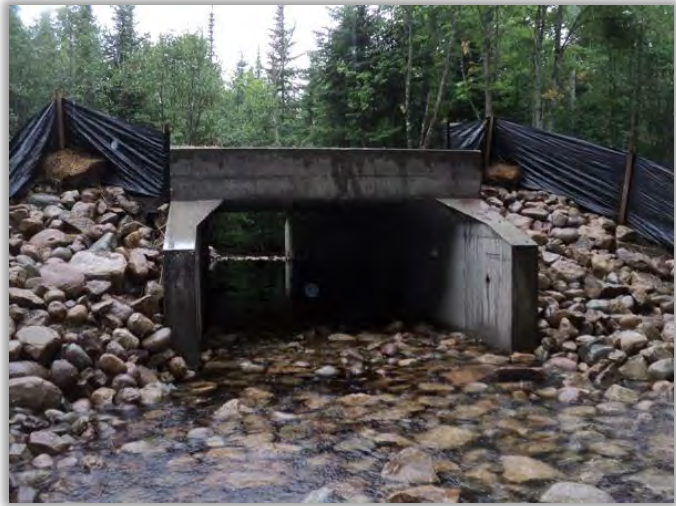
Figure 6-25 – Example of open bottom box culvert. Potential future solution @ 23 rd St crossing
