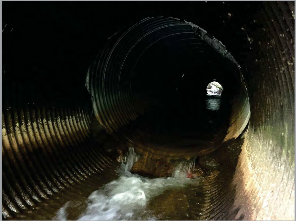
Figure 5-4 - 84-inch CMP culvert; Severe dislocations and significant deformation of pipe under roadway load. The forefront dislocation shown in this photograph is the location where a repair was completed on this culvert in 2011.
