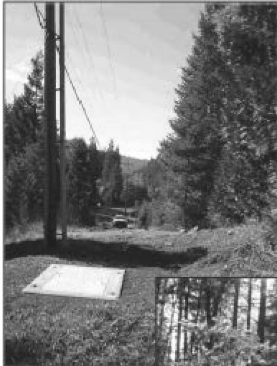
Top: Connection from overhead power to vault.
