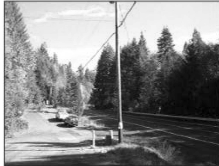
Right: Main power transmission line along Hwy. 126 and connection to underground (distant pole).
