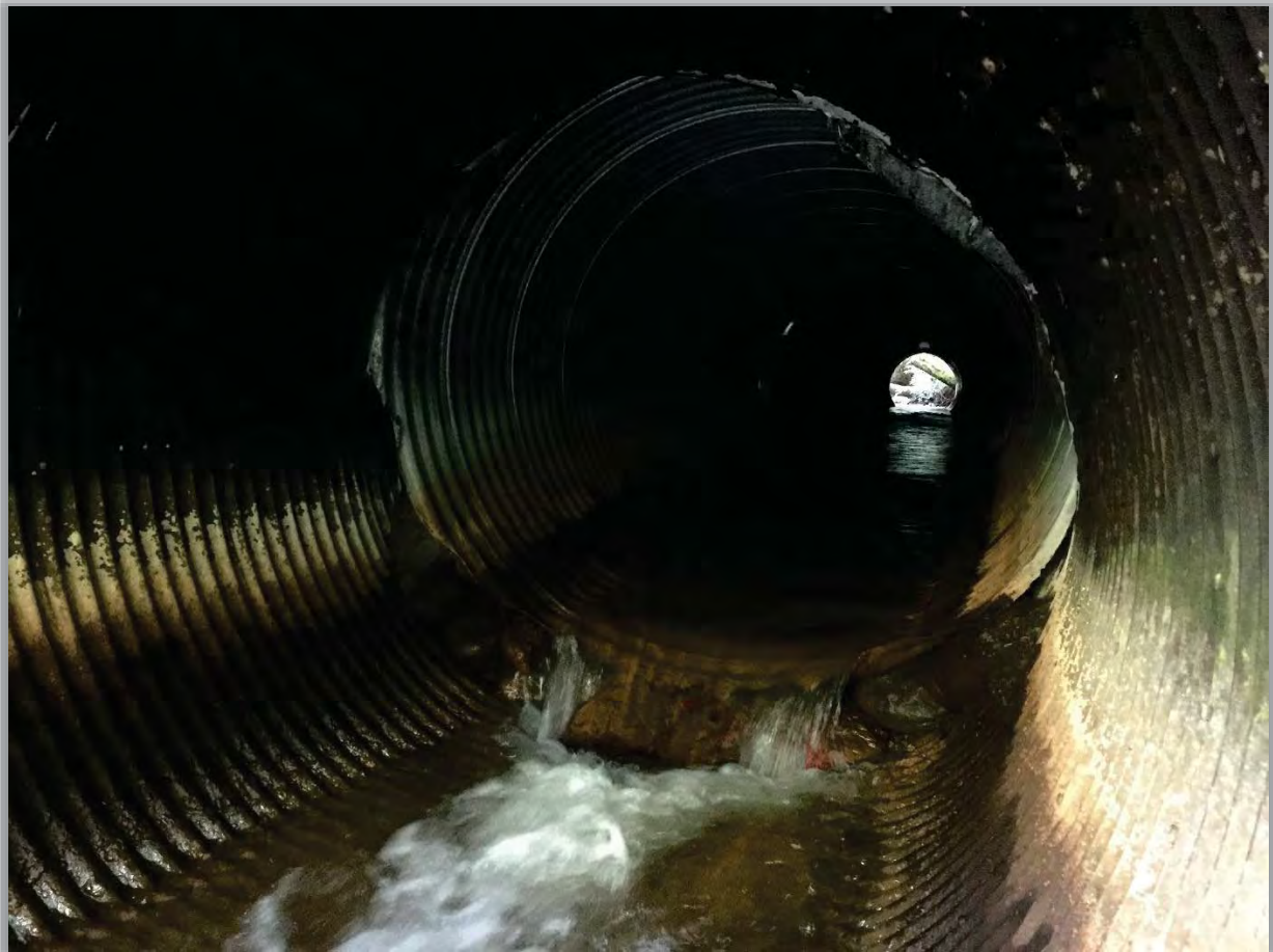
Figure 5-4 - 84-inch CMP culvert; Severe dislocations and significant deformation of pipe under roadway load. The forefront dislocation shown in this photograph is the location where a repair was completed on this culvert in 2011.
