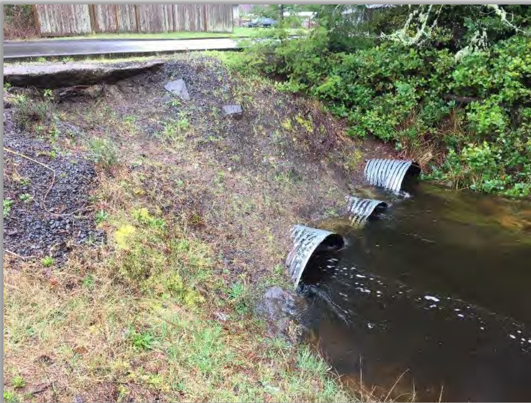
Figure 5-8 - Three 42-inch CMP culverts; insufficient capacity, roadside erosion
