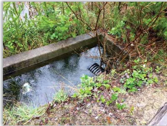
Figure 4-8 - Detention Ponds/ Weirs
