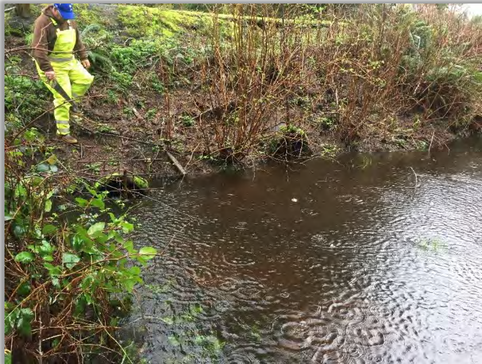
Figure 5-13 - Two 24-inch concrete culverts, one inactive, insufficient capacity
