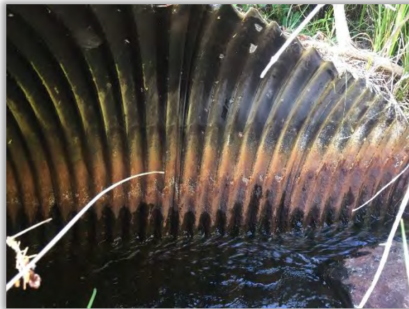
Figure 6-26 - Evidence of corrosion in existing pipe wall
