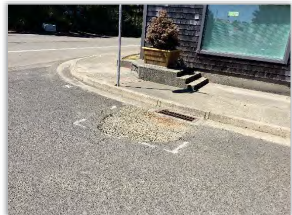
Figure 4-29 - Sinkhole on 18th St. caused by failed storm pipe
