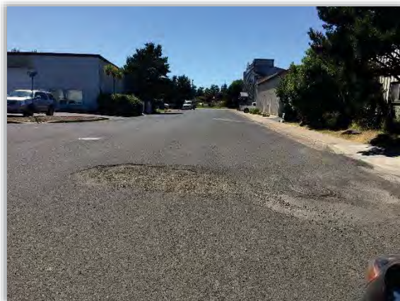
Figure 4-28 - Sinkhole on 18th St. caused by failed storm pipe
