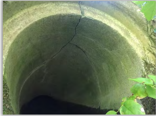
Figure 5-5 - 24-inch concrete outfall, cracking in the pipe crown
