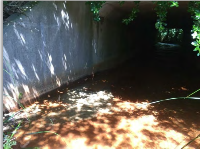
Figure 5-17 - 10' x 8' box culvert crossing Rhododendron Drive
