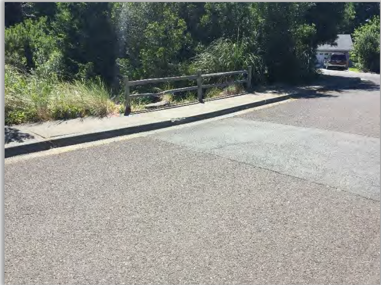
Figure 5-9 - Additional settlement has occurred after City trench patched with CLSM backfill
