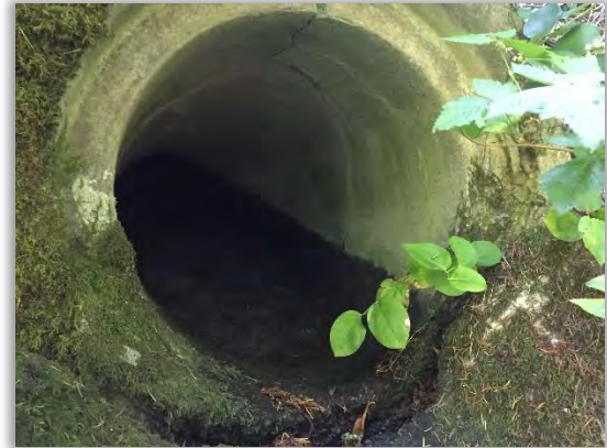
Figure 5-6 - Outfall pipe is sloped uphill in the direction of flow, causing sedimentation
