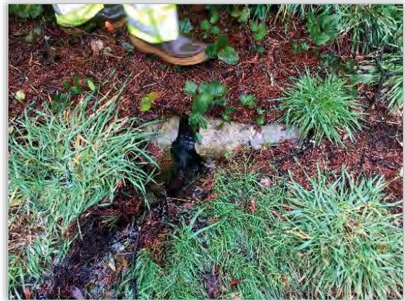
Figure 4-20 - Intentional break in 10" transite pipe for drainage
