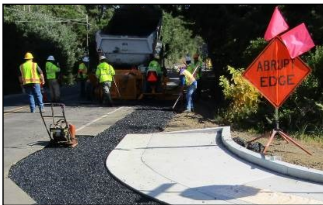
The base lift of permeable paving being installed for the Rhododendron Drive shoulder extension.
