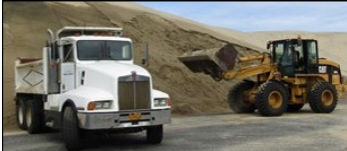
Removing sand from Oak Street that has drifted off the sand dune.
