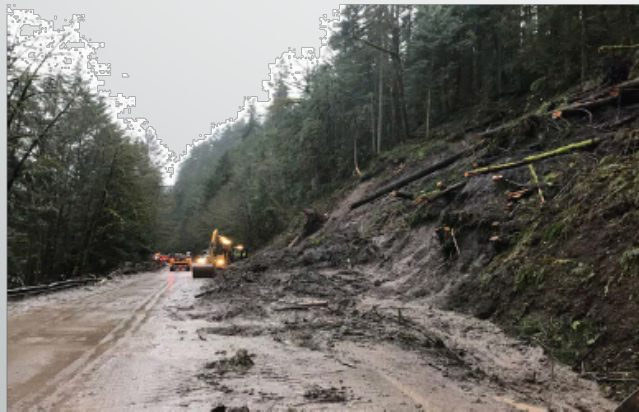
Rain induced landslide washing out portion of Highway 58 | via ODOT
