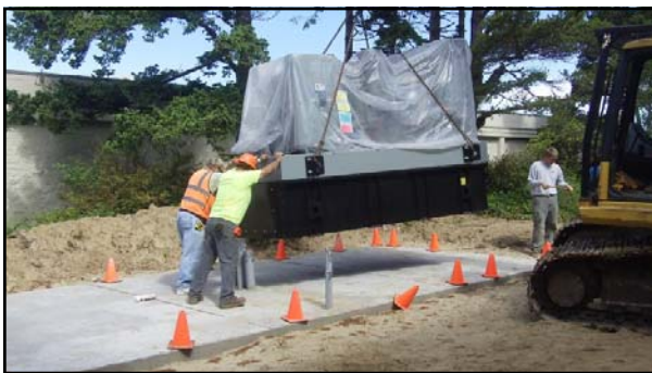
Public Works crews install an emergency generator outside of the Florence Events Center. The Friends of the FEC contributed $15,000 towards the project.
