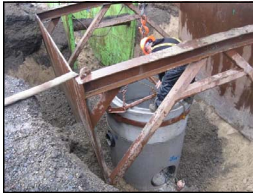
The City secured a zero interest loan in order to replace its existing trunk sewer line.
