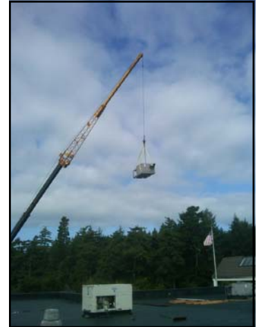
New HVAC units installed at the Justice Center will have a 25 to 30 year lifespan.
