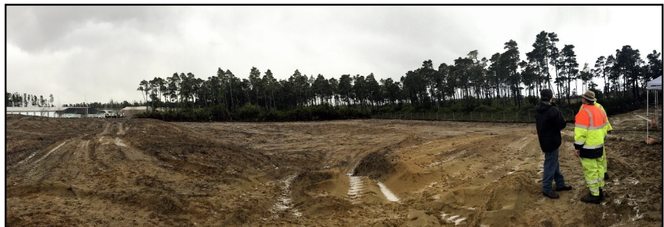
The 2.78-acre lot was cleared in December, and construction officially began on January 9, 2017.
