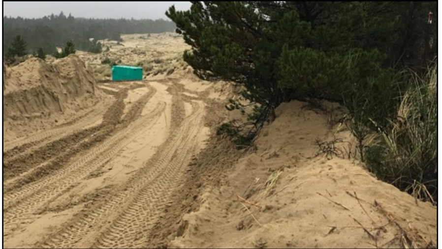
Access road being created to one of the wells. The green colored building is the well house that protects the electrical components of Well #8.
