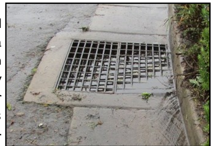
Close up of the 'bubble-up' catch basin with stormwater flowing out and down the street along the gutter.
