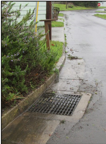
Stormwater flowing out of the 'bubble-up' catch basin at the corner of 2nd and Hwy 101. You can see the stormwater flowing down along the gutter towards Kingwood.
