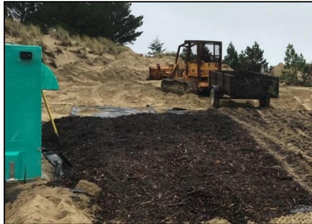
PW Crews creating a firm base at Well #8 for the well service rig.
