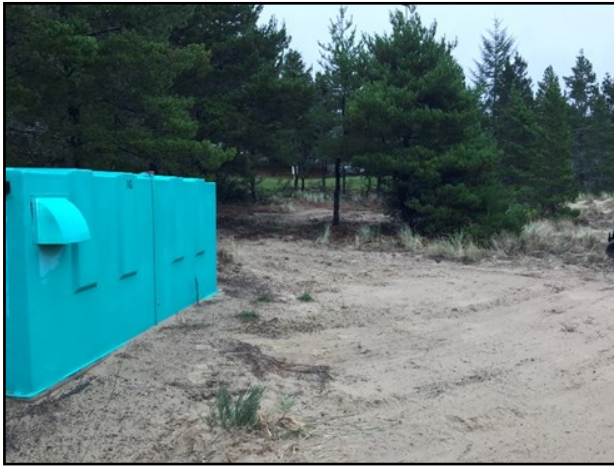
Well #10. Crews leveled out a spot in front of the well house for the service rig to set up.
