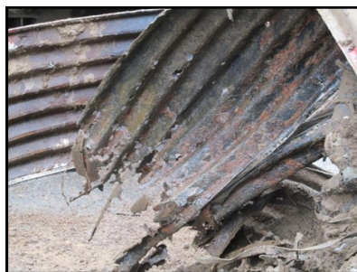
Public Works crews found that the entire length of the collapsed section of the culvert had deteriorated.
