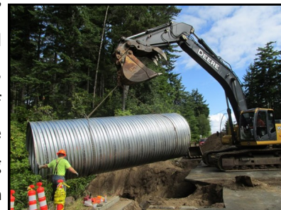
Ray Wells, Inc. completed the temporary repair of the culvert June 21st.
