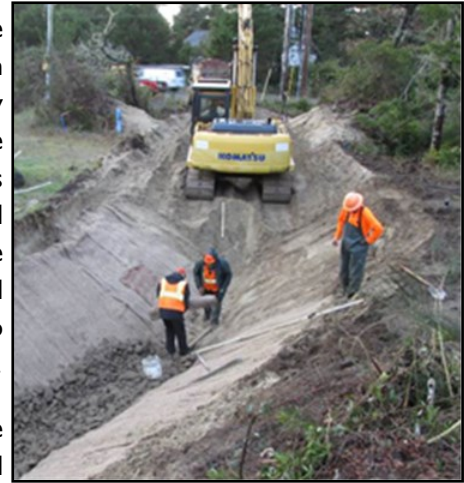
Crews from Ray Wells, Inc. installing jute mat along bottom of drainage swale.
