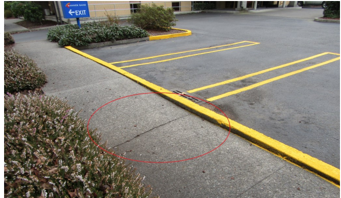
Example (circled in red) of a severe settlement resulting in an uneven sidewalk and tripping hazard.
