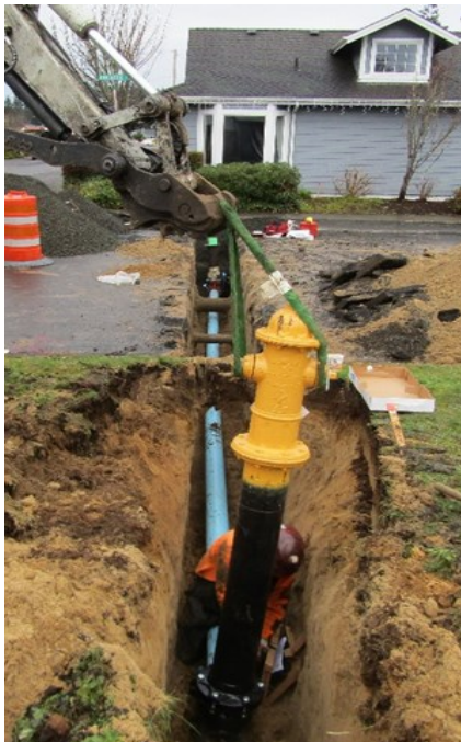
Setting new fire hydrant at the southwest corner of Rhododendron and Kingwood.
