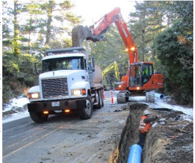
Carter & Company installing the new 16-inch water main on Rhododendron Drive in a dusting of snow.
