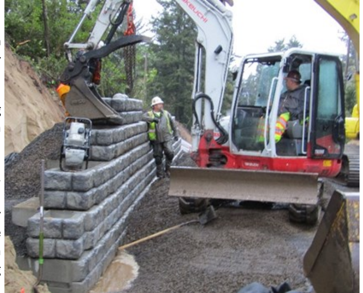
Installing gravity block retaining wall on the south side of Rhododendron Drive.
