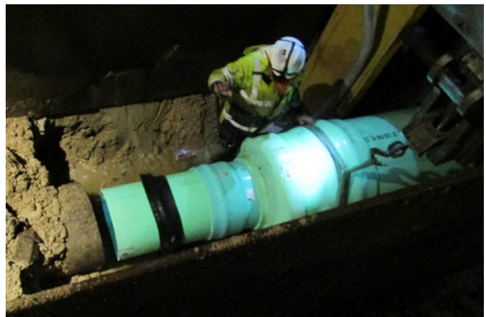
Connecting the new 36-inch PVC stormwater pipe to the existing 24-inch concrete pipe. Installing the crossing now eliminates the need to excavate Rhododendron Drive in the future.
