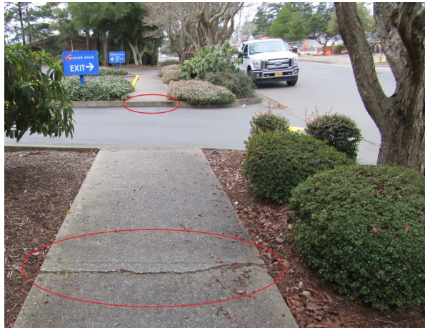
What's wrong with this? Circled in red (bottom of photo) is a vertical separation of more than ¼-inch. The circled area towards the top of the photo is the drop off/step up creating a barrier to pedestrian traffic since there is not a ramp.
