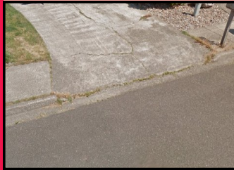
Uneven Slopes & Curbs
