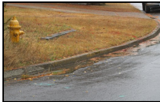
Stormwater Not Draining
