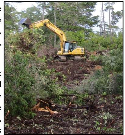
Ray Wells, Inc. excavator clearing vegetation and root mat from the new PW Operations Facility.
