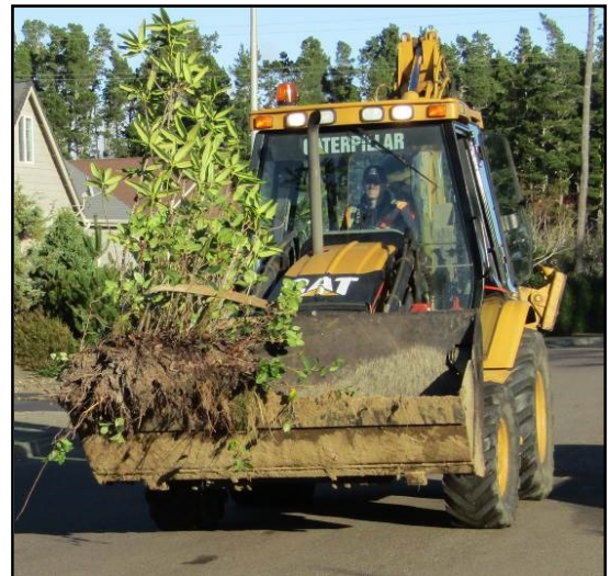
PW staff transporting a large rhododendron that was salvaged from the site.
