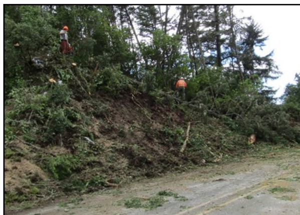
Contractor's crews clearing the trees and vegetation on the south side of Rhododendron adjacent to the wastewater treatment plant. This is the location of one of the retaining walls.
