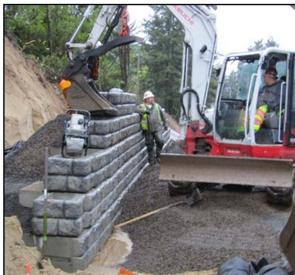
Installing the first of three gravity block retaining walls. This one is on the south side of Rhododendron Drive.
