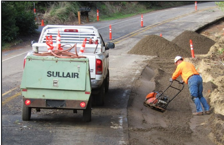
Contractor extending the shoulder of Rhododendron Drive west of the entrance to the hospital for a new bike lane and sidewalk.
