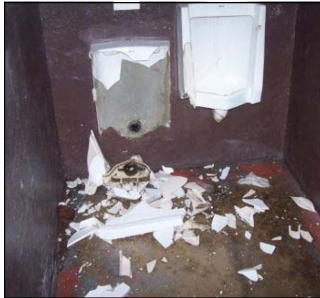
Damage to the Miller Park restrooms on March 19th will cost City taxpayers approximately $3,600 to repair and forced the City to close the facilities indefinitely.
