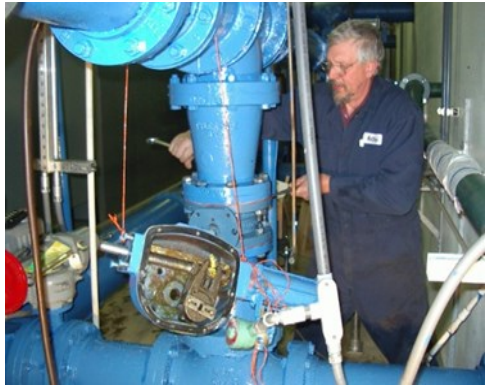
Photo to left is of one of our highly trained and skilled plant operators performing a repair of a malfunctioning control valve at the water treatment plant.
